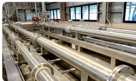
Piping system II (Maximum diameter is 300mm)
